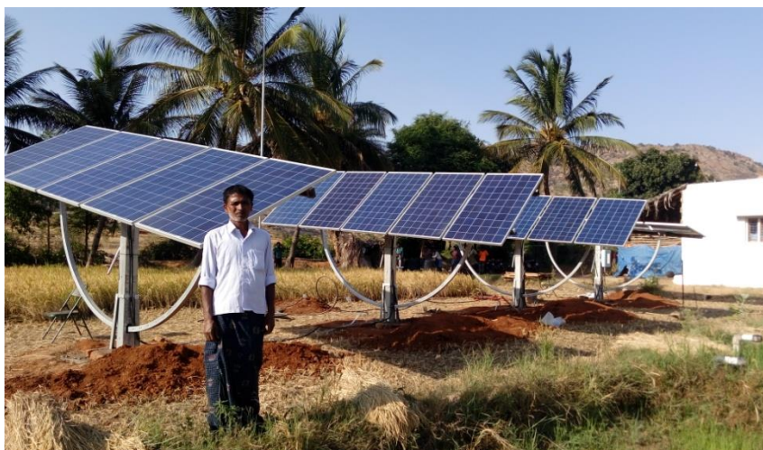
Fig. 1: Solar PV powered water pumping system
